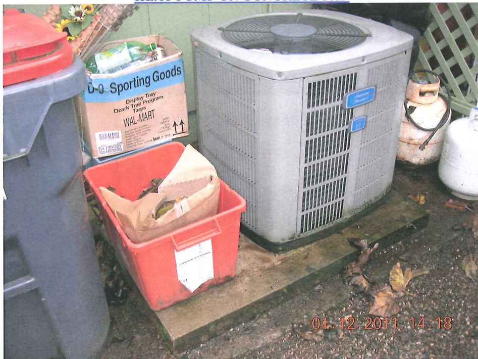
HEAT PUMP ON CONCRETE PAD
