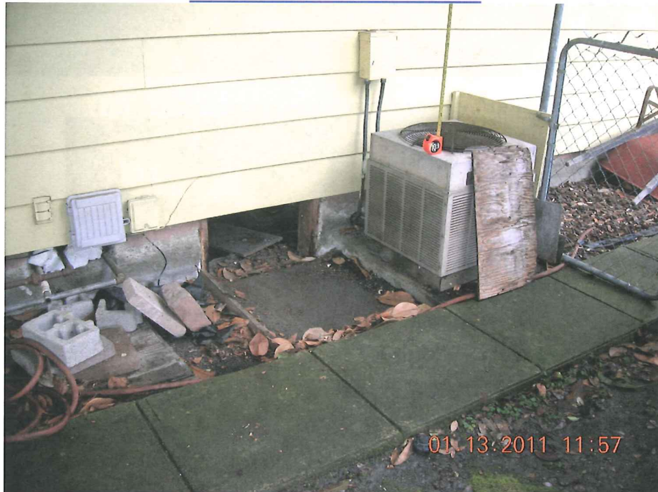
HEAT PUMP ON CONCRETE PAD
