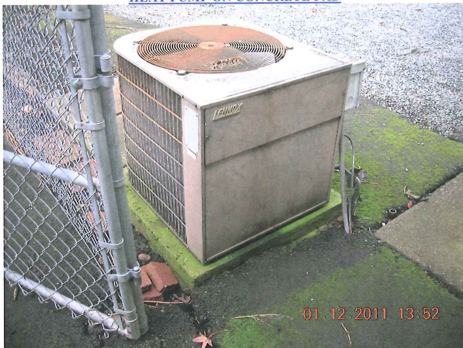
HEAT PUMP ON CONCRETE PAD
