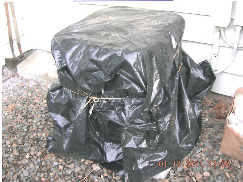
HEAT PUMP ON CONCRETE PAD
