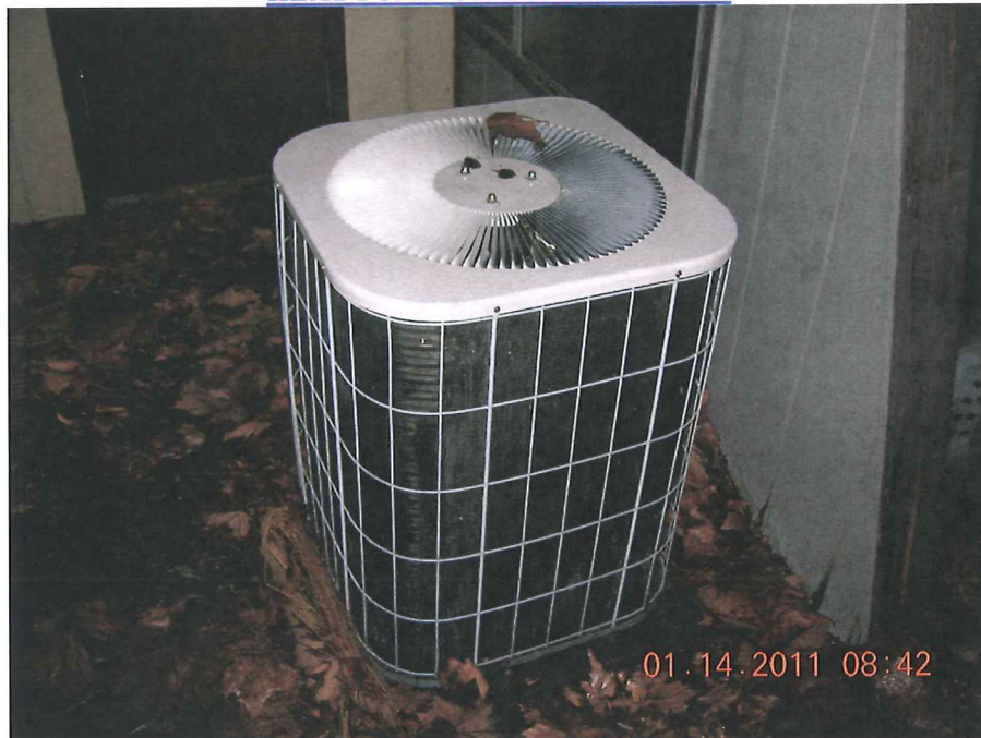
HEAT PUMP ON CONCRETE PAD
