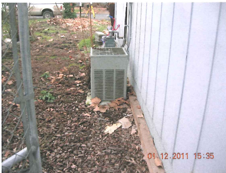
HEAT PUMP ON CONCRETE PAD
