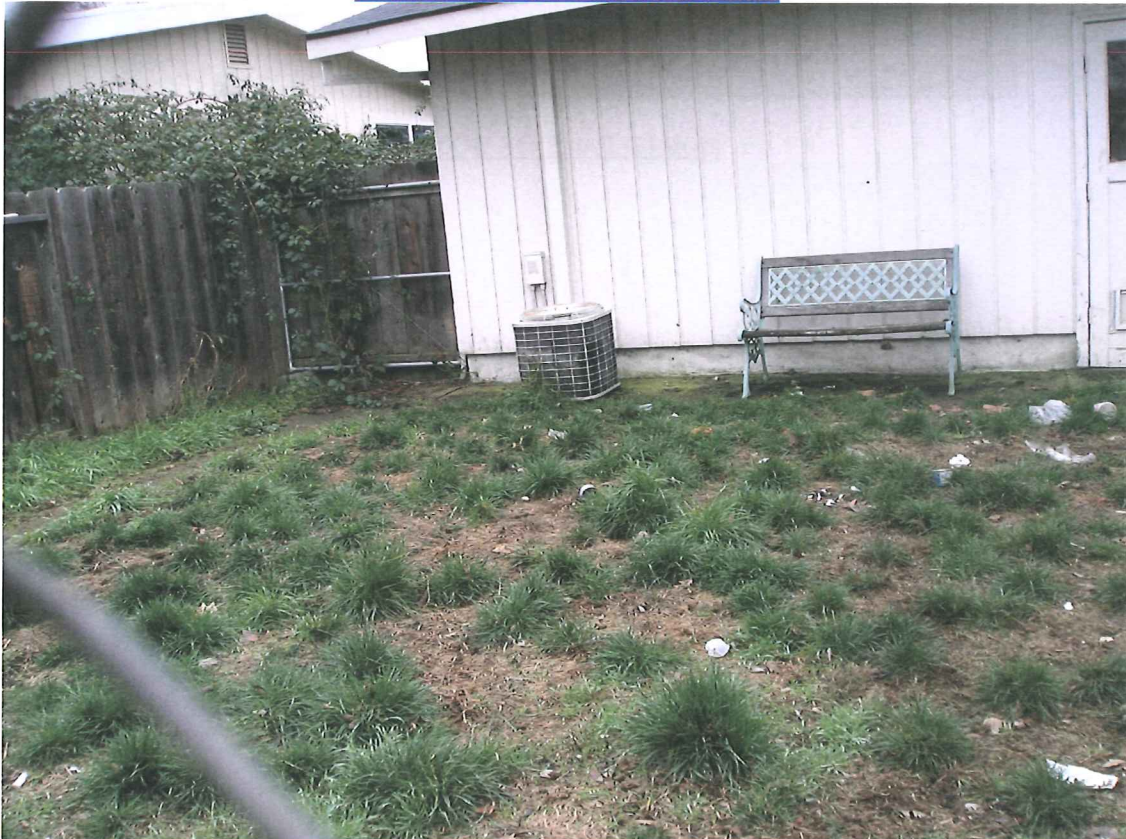
HEAT PUMP ON CONCRETE PAD
