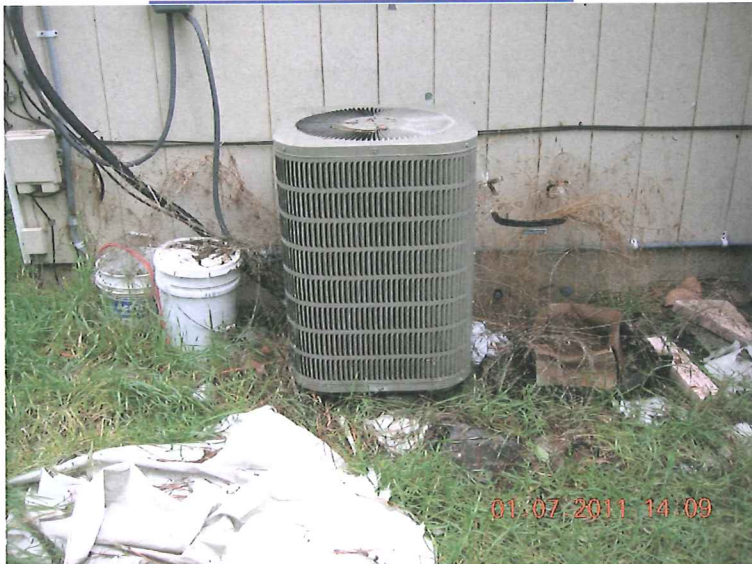
HEAT PUMP ON CONCRETE PAD
