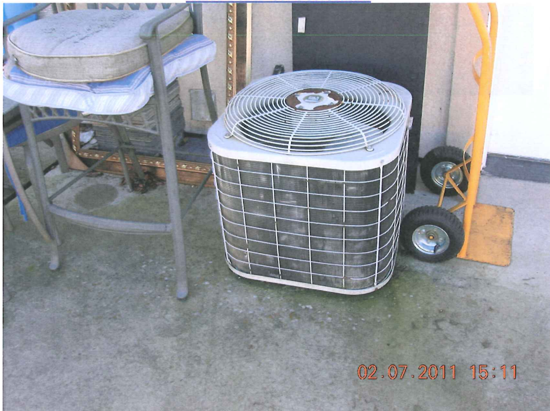
HEAT PUMP ON CONCRETE
