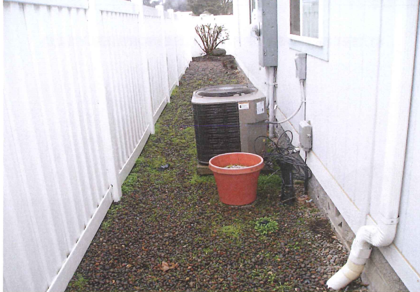
HEAT PUMP ON CONCRETE PAD (LOOKING SOUTHERLY ALONG EASTELRY WALL)
