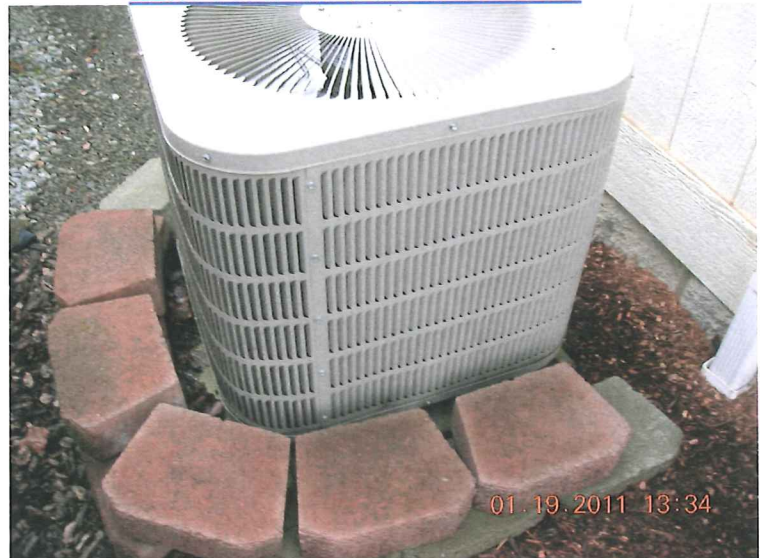
HEAT PUMP ON A CONCRETE PAD
