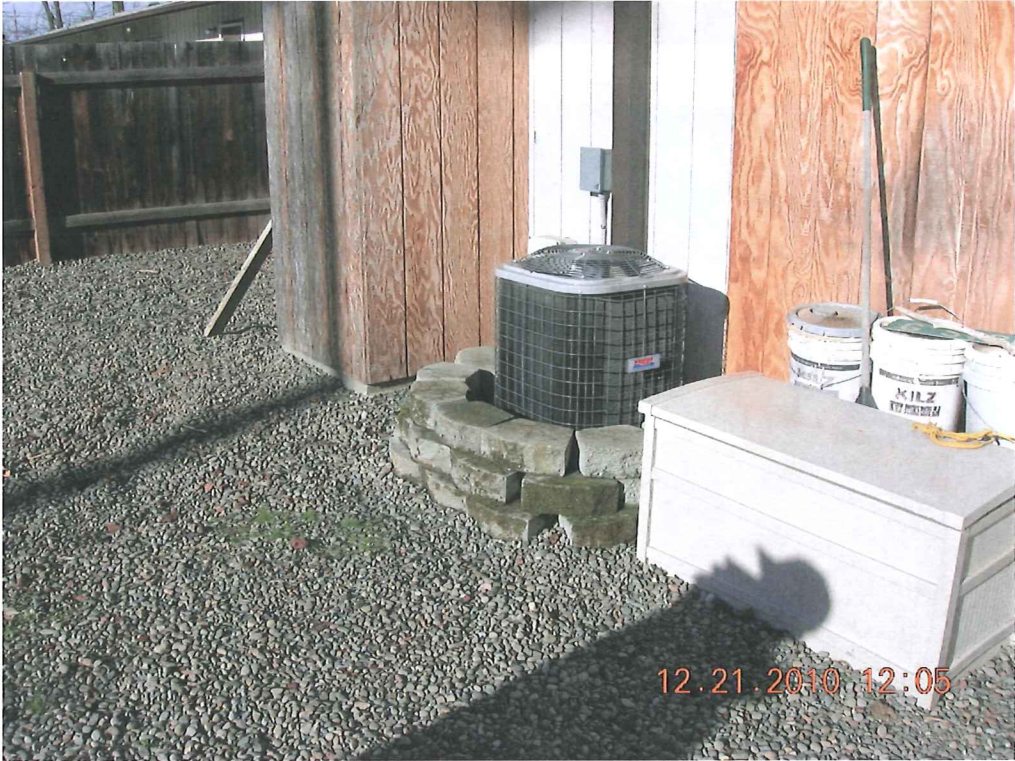
HEAT PUMP ON CONCRETE PAD
