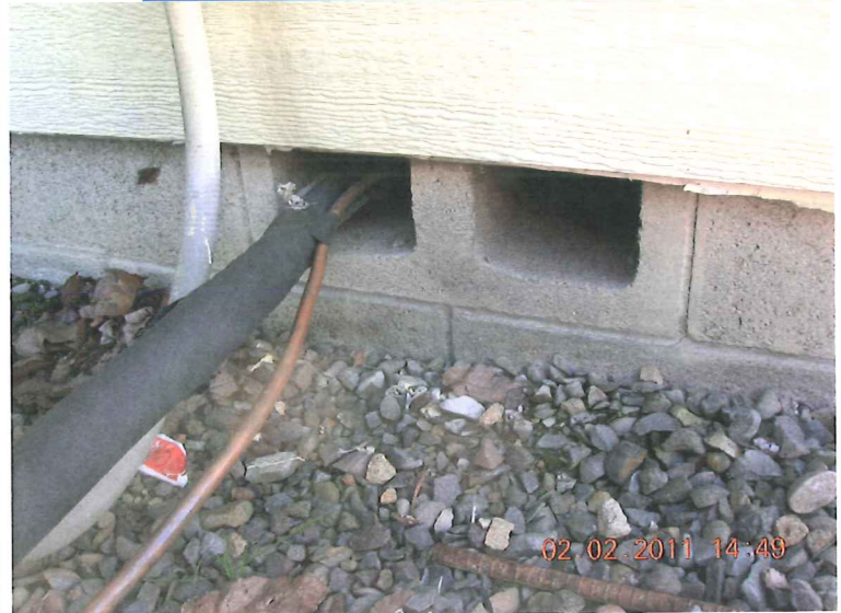
CMU BLOCK FOUNDATION VENT (8)
