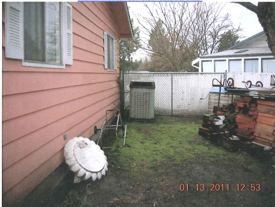
HEAT PUMP ON CONCRETE PAD
