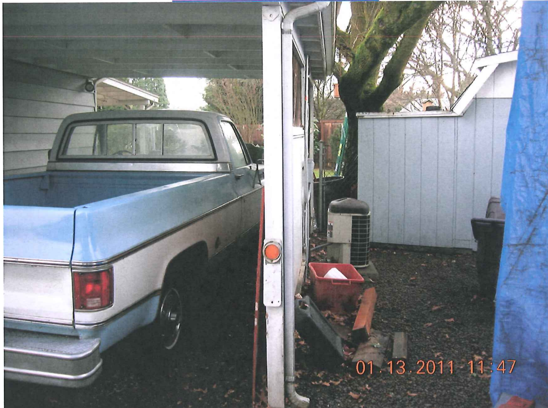
HEAT PUMP ON CONCRETE PAD
