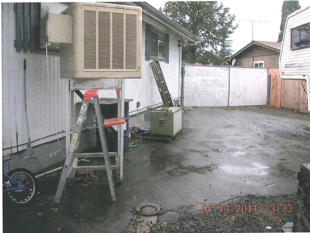
SWAMP-COOLER ON A STAND AND A HEAT PUMP ON CONCRETE PAD (IN THE BACKGROUND)
