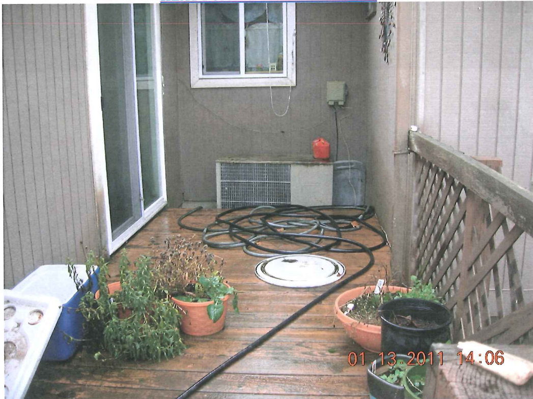
HEAT PUMP ON CONCRETE PAD
