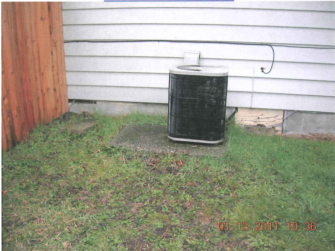
HEAT PUMP ON CONCRETE PAD
