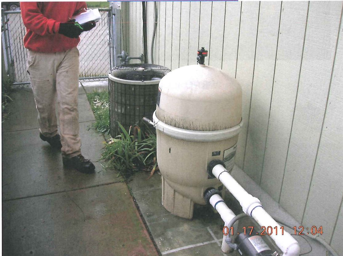
HEAT PUMP ON CONCRETE PAD
