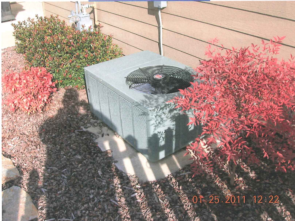
HEAT PUMP ON CONCRETE PAD
