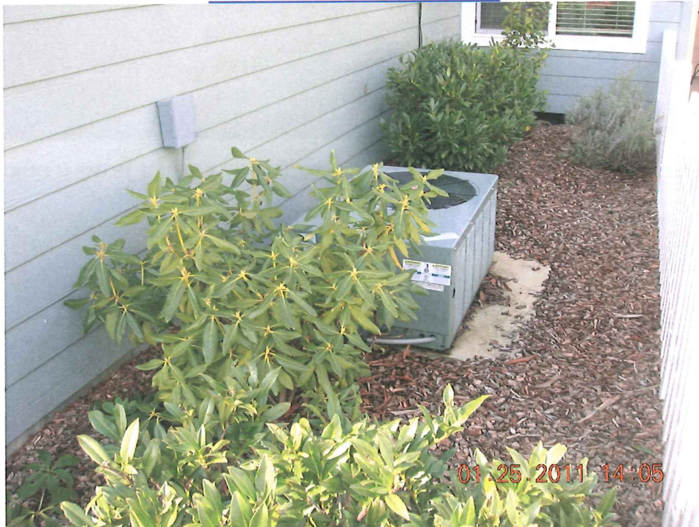
HEAT PUMP ON CONCRETE PAD
