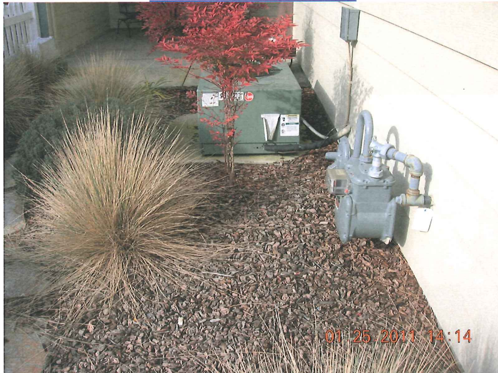
HEAT PUMP ON CONCRETE PAD
