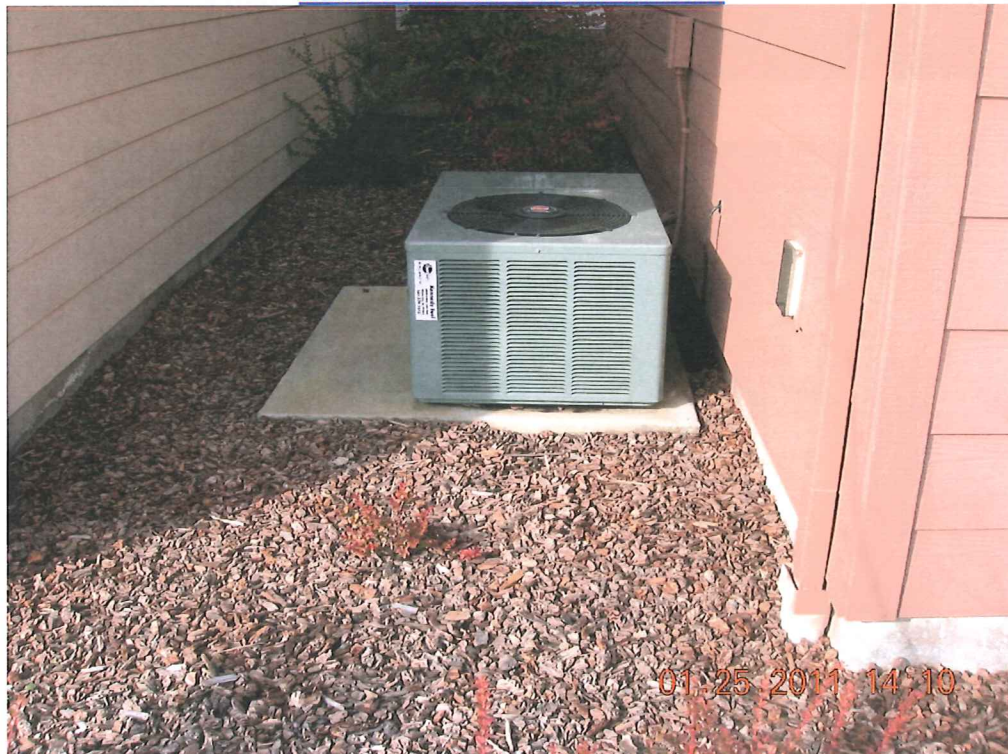
HEAT PUMP ON CONCRETE PAD
