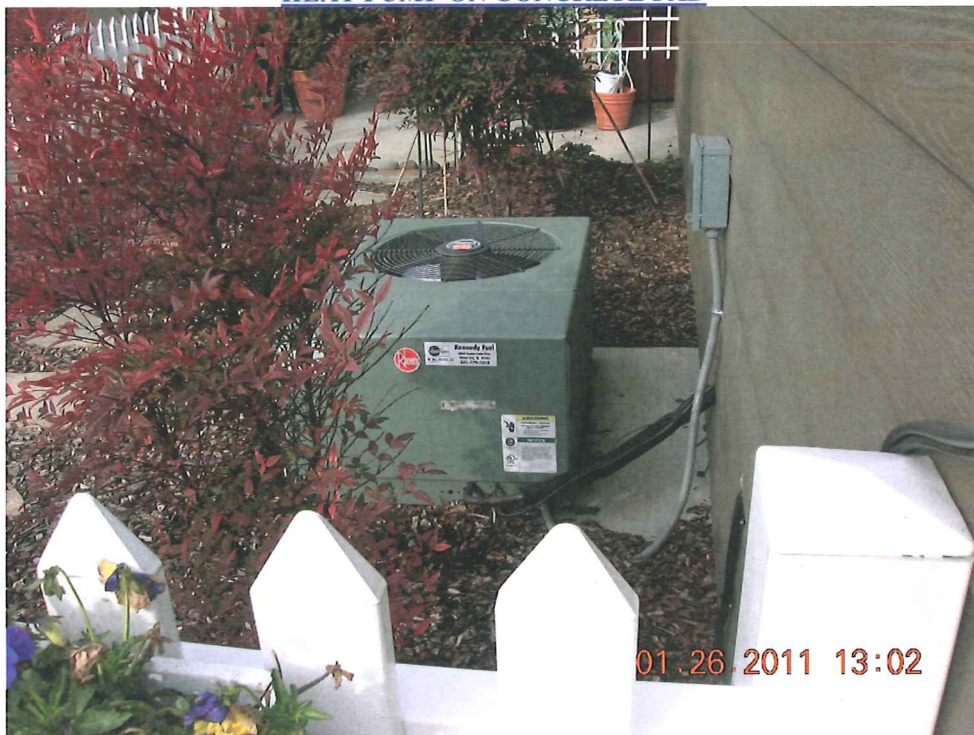
HEAT PUMP ON CONCRETE PAD
