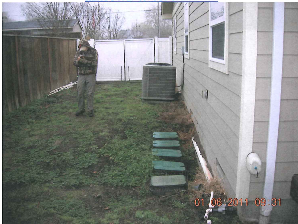
HEAT PUMP ON CONCRETE PAD
