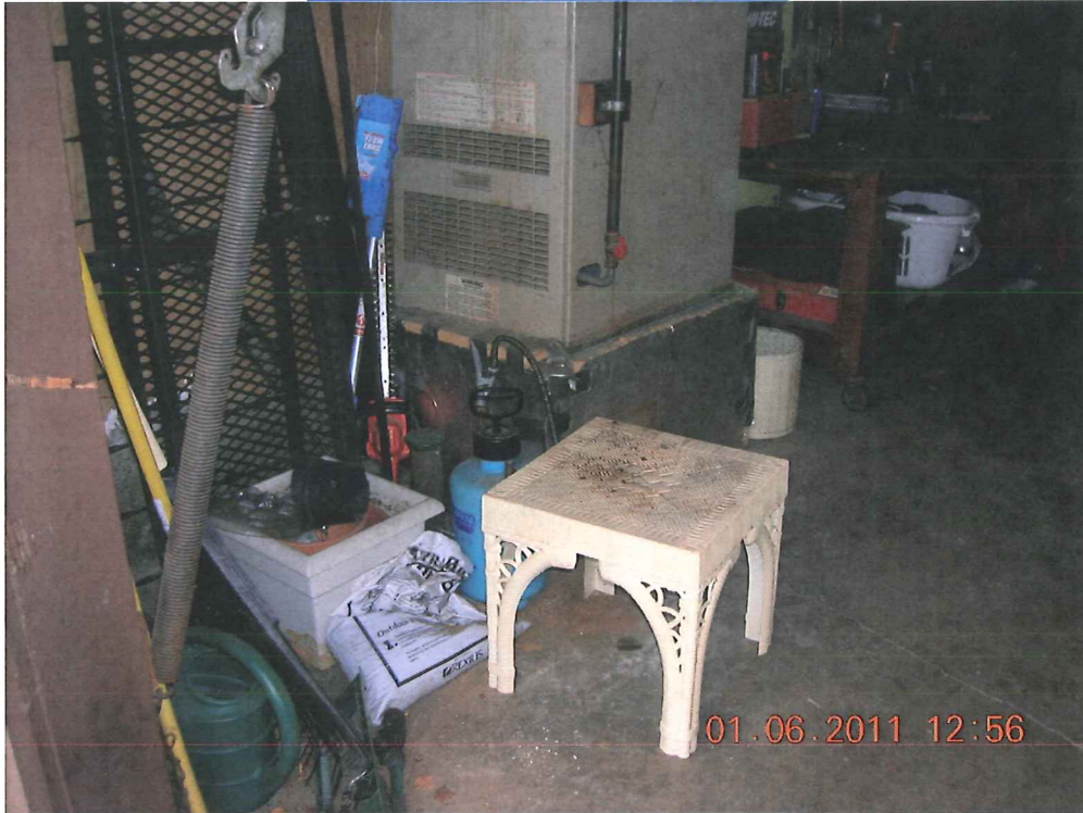
ELEVATED FURNACE IN GARAGE
