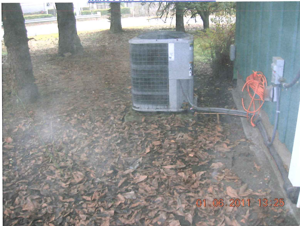
HEAT PUMP ON CONCRETE PAD
