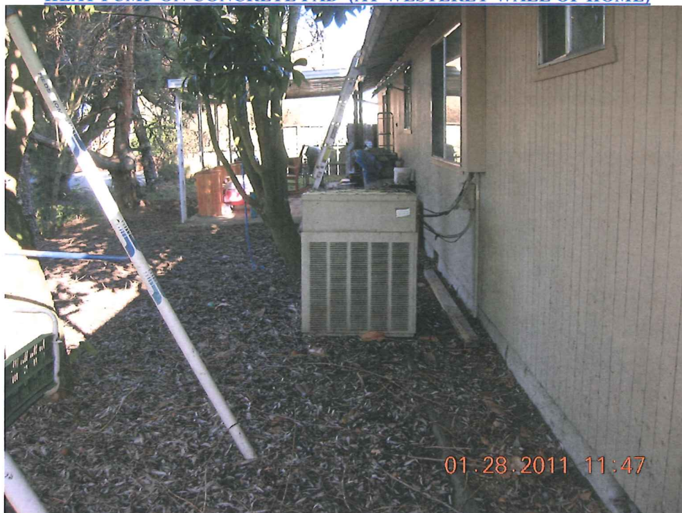
HEAT PUMP ON CONCRETE PAD (AT WESTERLY WALL OF HOME)
