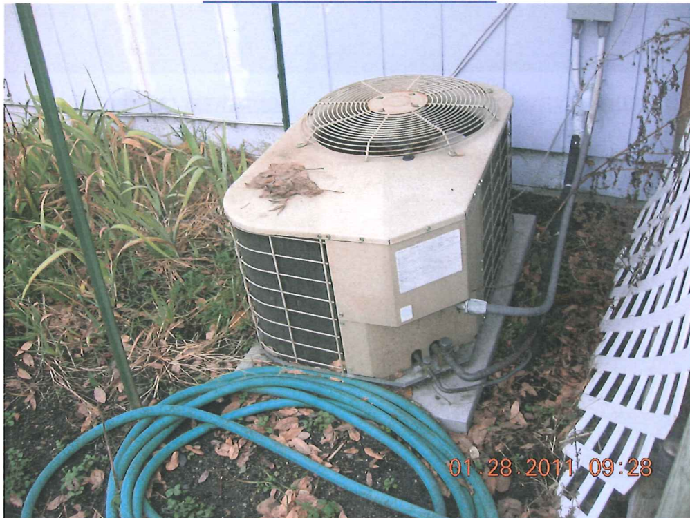
HEAT PUMP ON CONCRETE PAD
