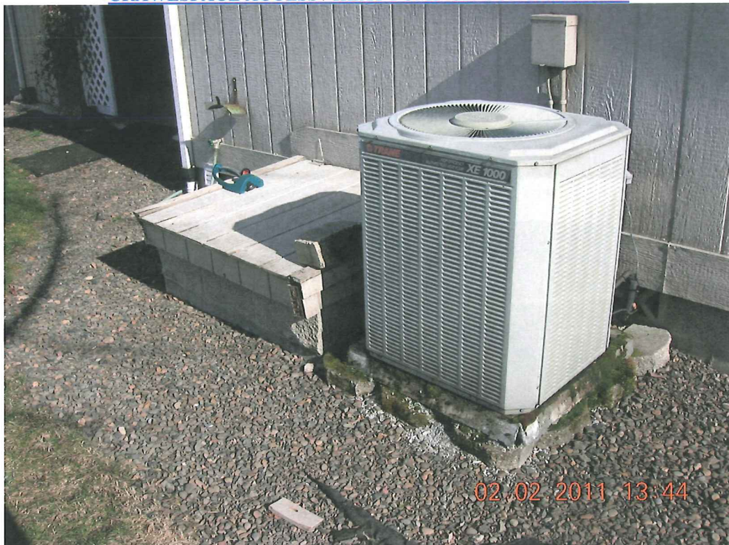
CRAWLSPACE ACCESS / HEAT PUMP ON CONCRETE PAD
