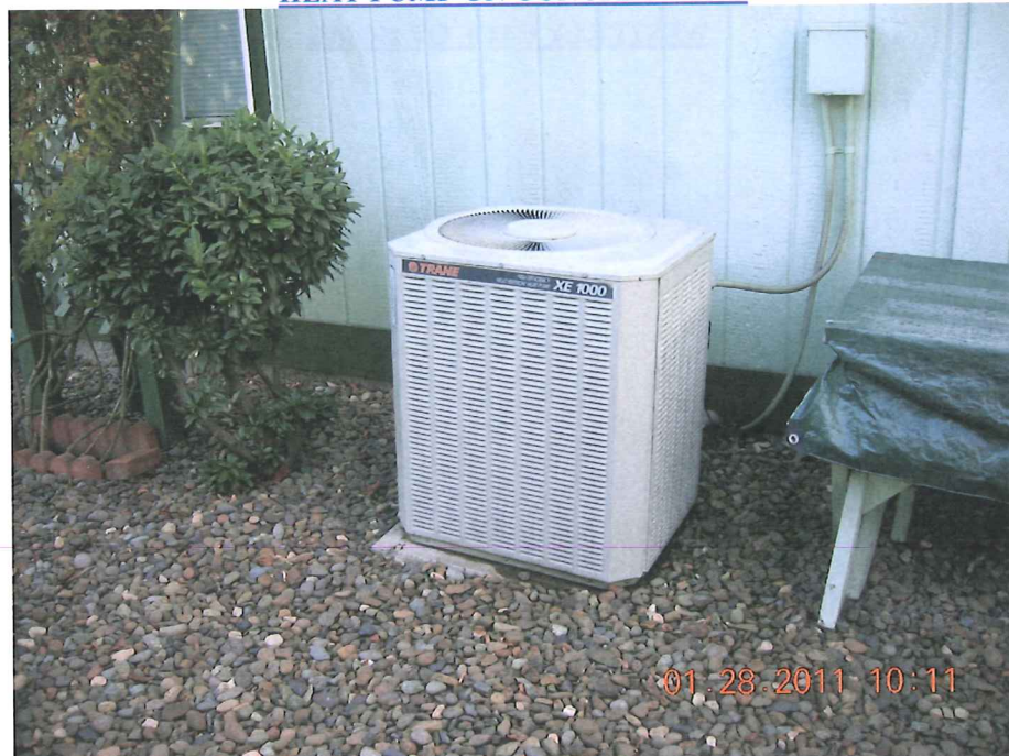
HEAT PUMP ON CONCRETE PAD
