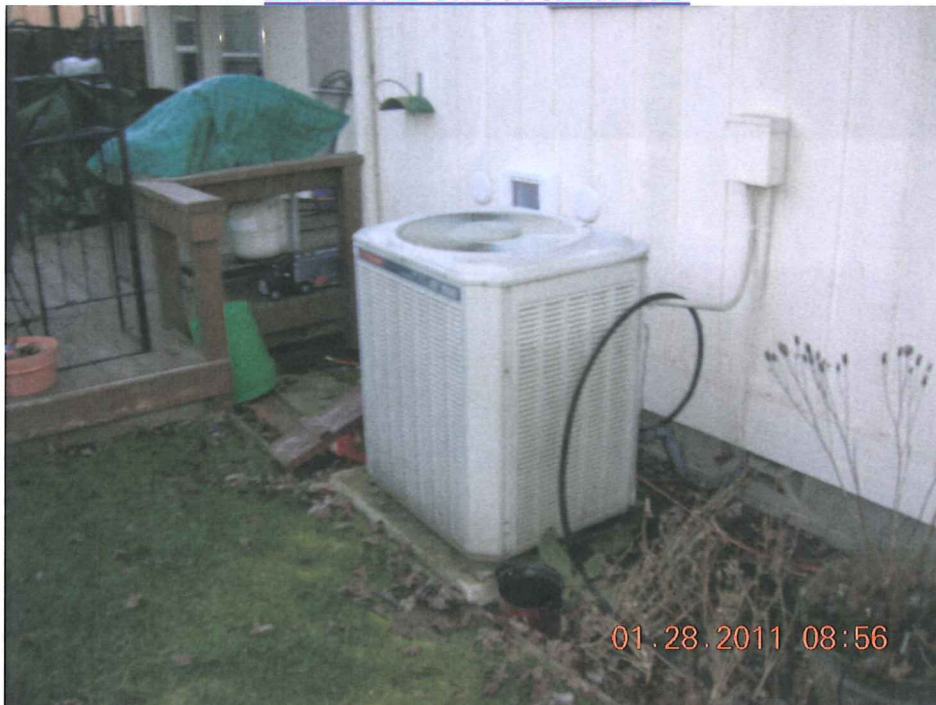
HEAT PUMP ON CONCRETE PAD
