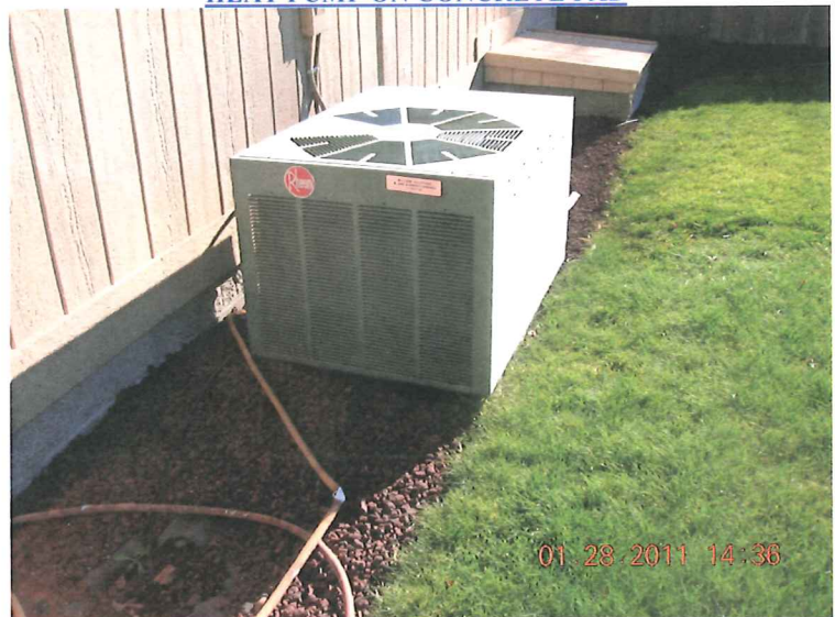
HEAT PUMP ON CONCRETE PAD
