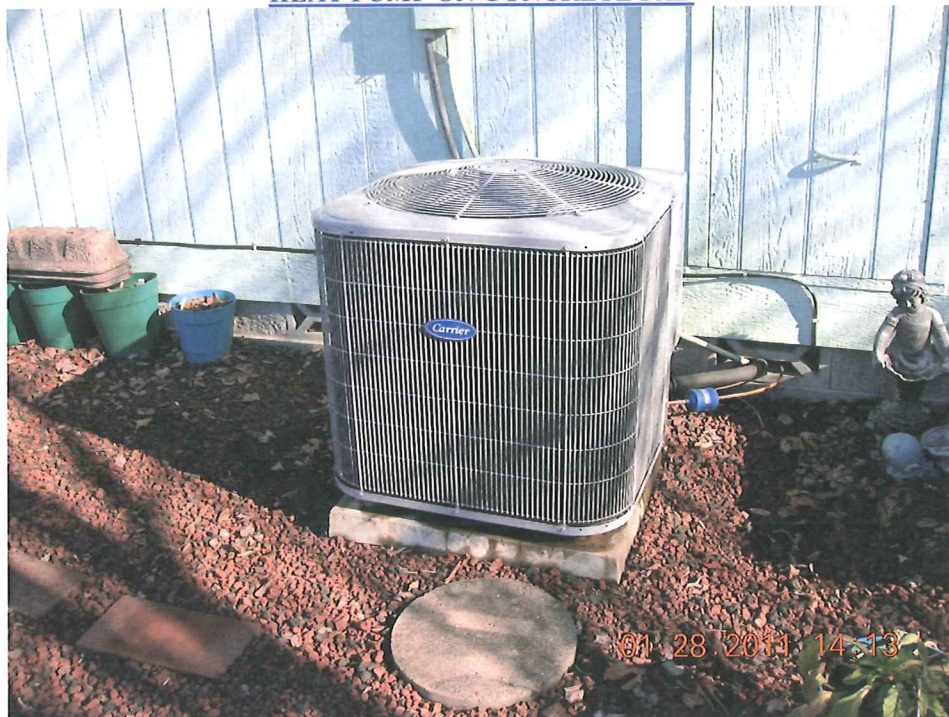
HEAT PUMP ON CONCRETE PAD
