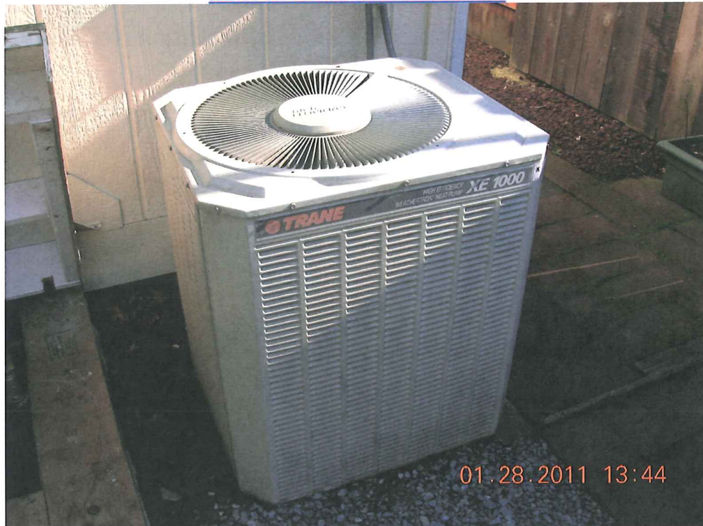
HEAT PUMP ON CONCRETE PAD
