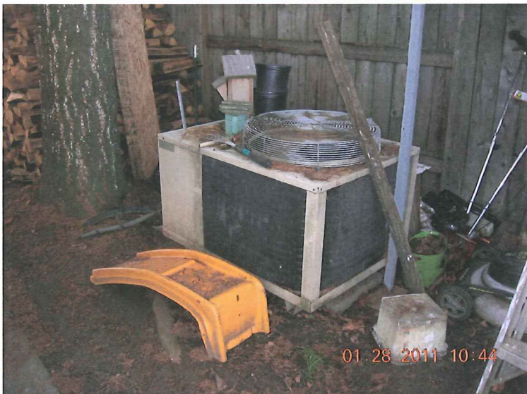
HEAT PUMP ON CONCRETE BLOCKS
