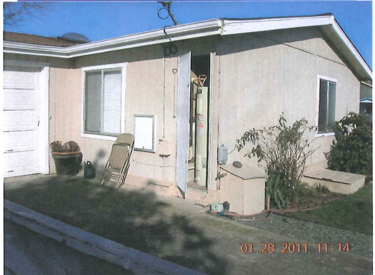
WATER HEATER AT SOUTHEAST CORNER OF HOME
