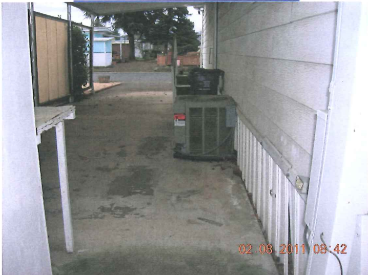
HEAT PUMP ON CONCRETE SLAB
