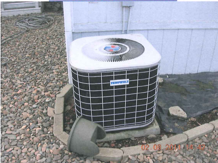
HEAT PUMP ON CONCRETE PAD
