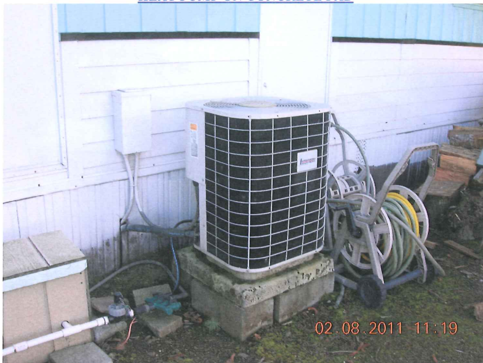
HEAT PUMP ON CONCRETE PAD
