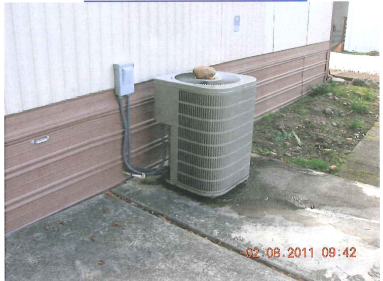
HEAT PUMP ON CONCRETE SLAB
