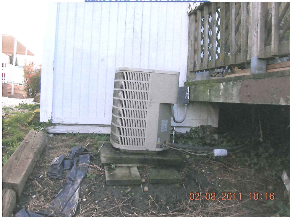
HEAT PUMP ON CONCRETE PAD
