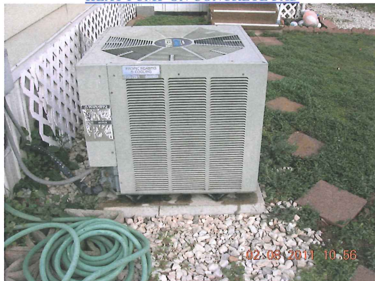
HEAT PUMP ON CONCRETE PAD
