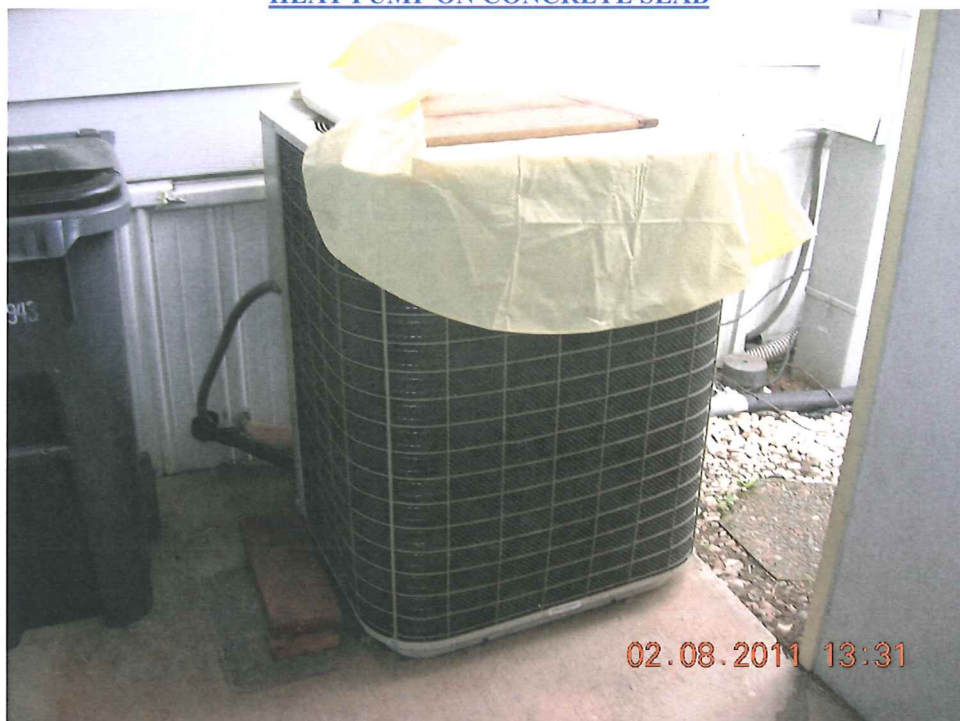
HEAT PUMP ON CONCRETE SLAB
