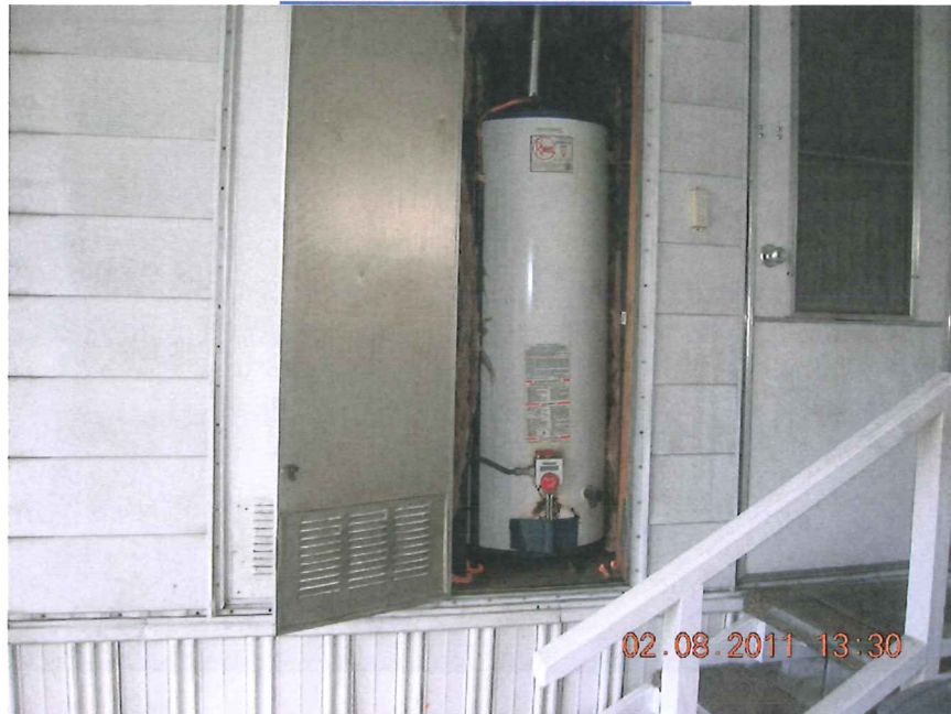
ELEVATED WATER HEATER
