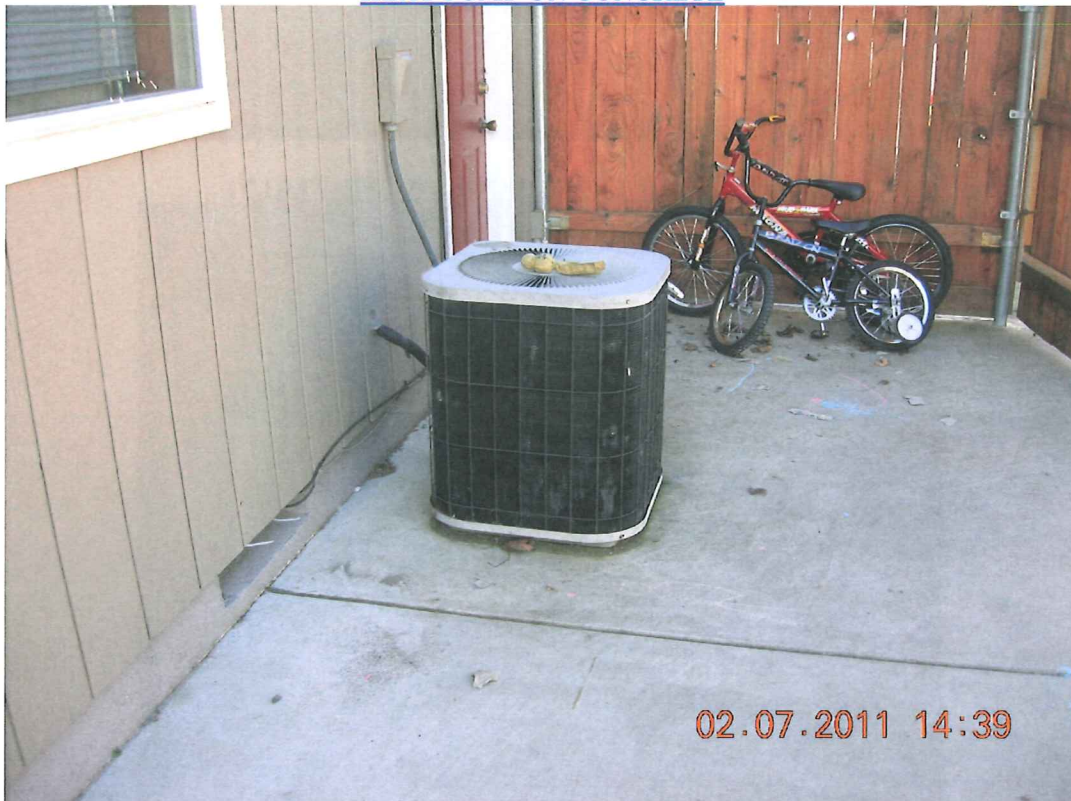
HEAT PUMP ON CONCRETE
