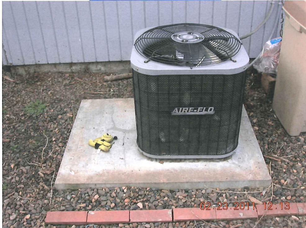
HEAT PUMP ON CONCRETE PAD
