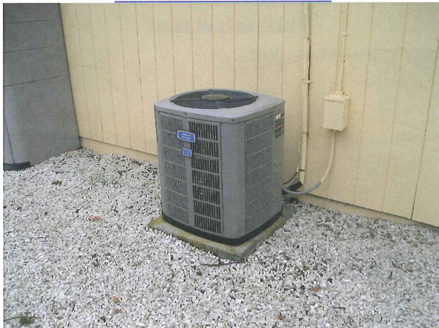
HEAT PUMP ON CONCRETE PAD
