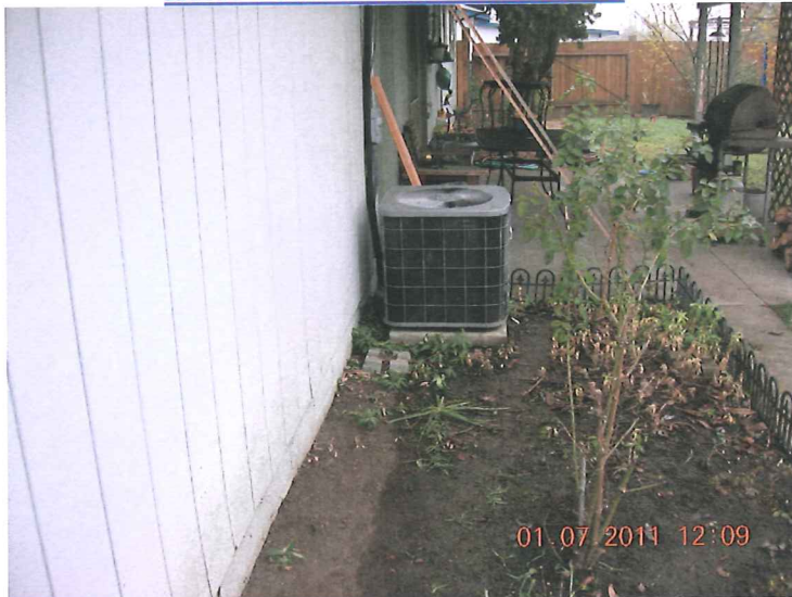
HEAT PUMP ON CONCRETE PAD
