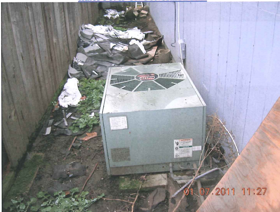
HEAT PUMP ON CONCRETE PAD
