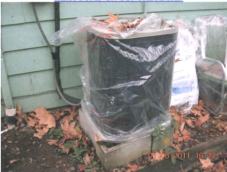
HEAT PUMP ON CONCRETE PAD
