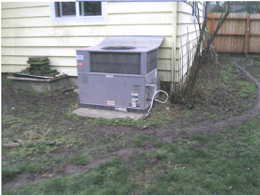
HEAT PUMP ON CONCRETE PAD
